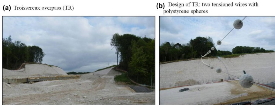
FIGURE 3 Pictures of bat overpass temporarily installed during road construction on road D901 (TR) (a, b) to the north of Paris
